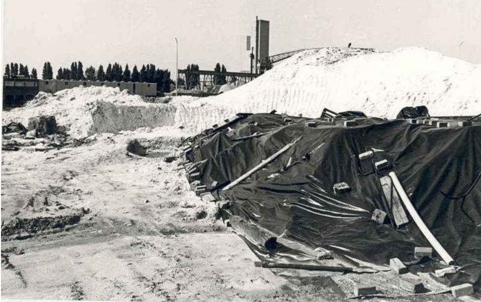
Photo 1. This photo was taken during the excavation of the waste HCH isomers in the eastern Netherlands to be shipped for disposal at German salt mines.
